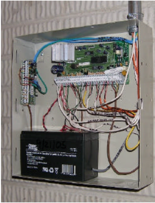
The installer of this system marked the battery so the next technician will know how old it is.
